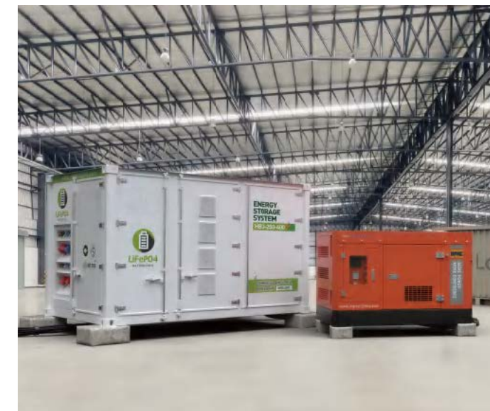
Power Bank &amp; DG
