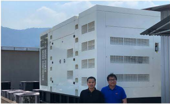
Honduras, Cummins, Standby
